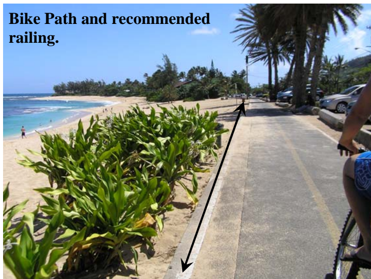
Bike Path Undermining and drop off
